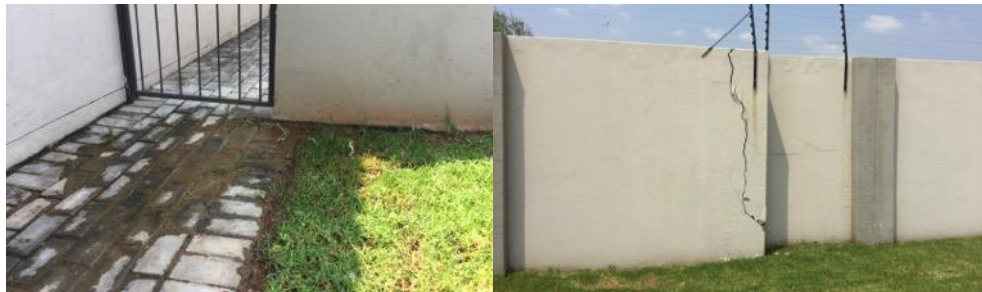
Induced interflow and poor drainage
